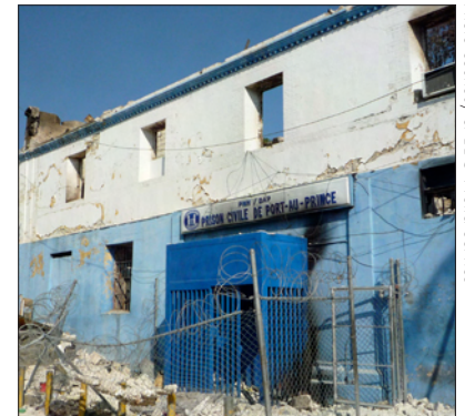
Haiti's largest penitentiary, the Prison Civile, was badly damaged in the January 2010 quake.
